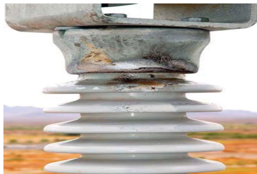
FIG.1: Flashed 230 KV Porcelain Insulator
